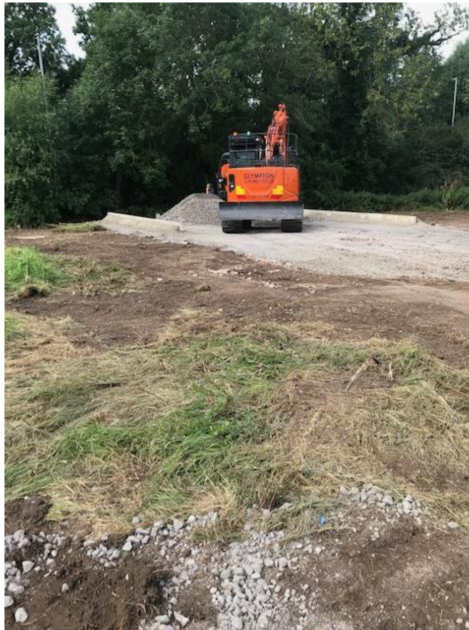
Figure 2 – Hardstanding in the process of being laid at the main site entrance, from High Street.
