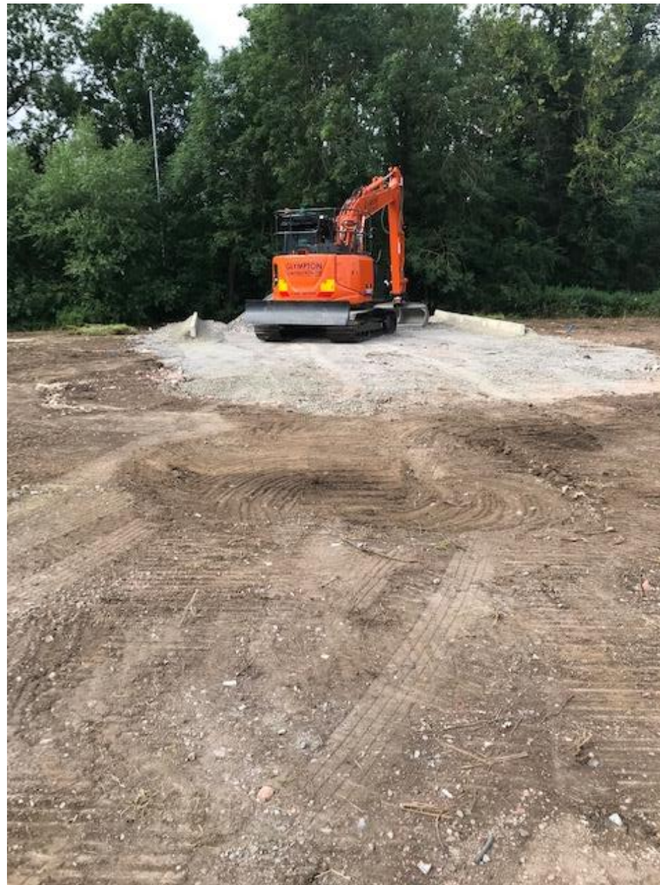
Figure 3 – Hardstanding in the process of being laid at the main site entrance, from High Street.
